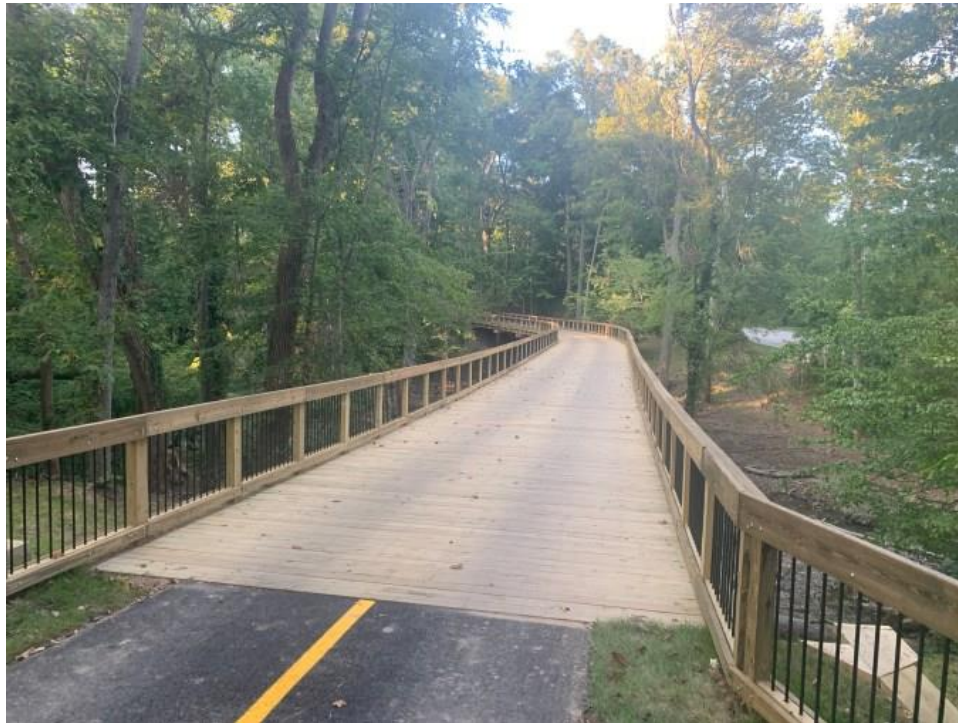
Figure 12. Recently Reconstructed Bridge 12 near Fort Hunt Park Source: Friends of Mount Vernon Trail 2023
